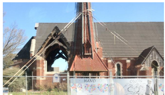
Earthquake damaged church
